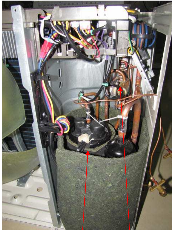
Internal view (compressor, 4 way valve)
